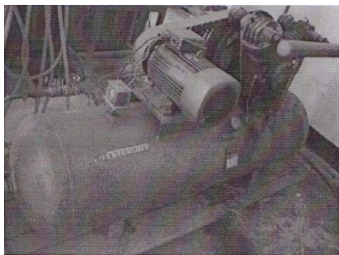
Figure 3.6: Photograph of Air Compressor
