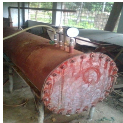
Figure 3.7C: photograph of pressure treating chamber.
